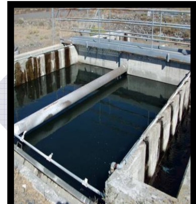
Large Imhoff Tank
