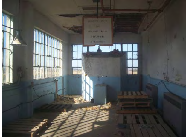
Surveillance Workshop (failing roof & insulation)
