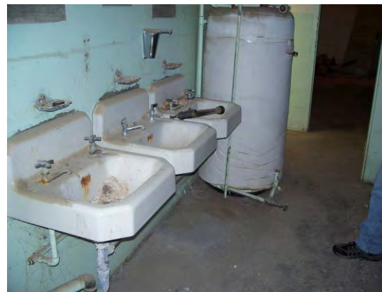
Plumbing Code Violation- Building 11
