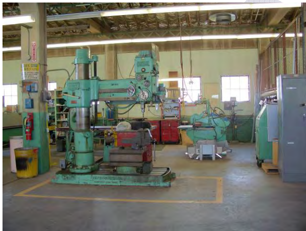
Maintenance Shop Machines
