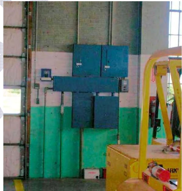
Old Main Breaker and Distribution Panel Eastside
