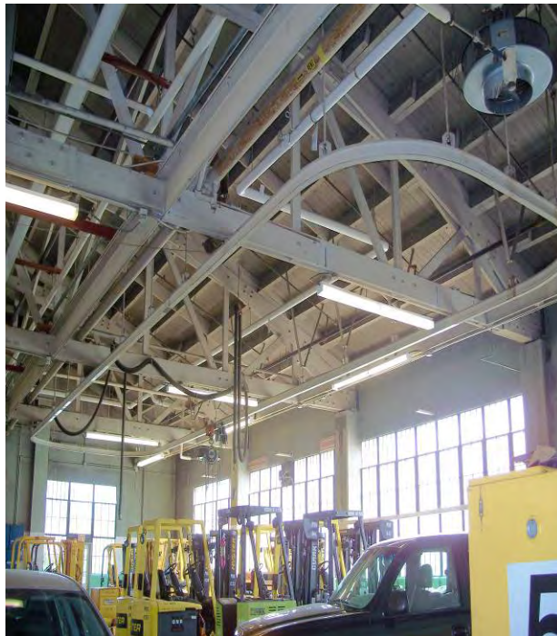
Monorail Hoists for Servicing Vehicles
