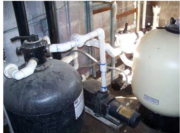
Pool Pumping & Filtration System
