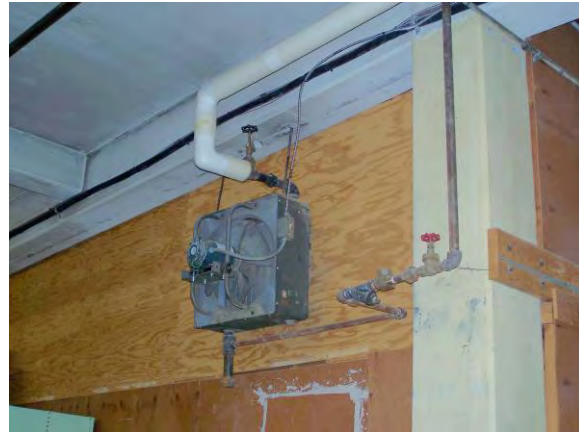
Typical: Admin Area Steam Unit Heater
