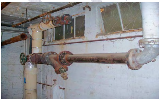
Piping Code Violation- Building 11 Basement
