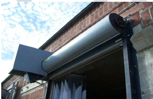
Building Motorized Roll-up Door (unused)
