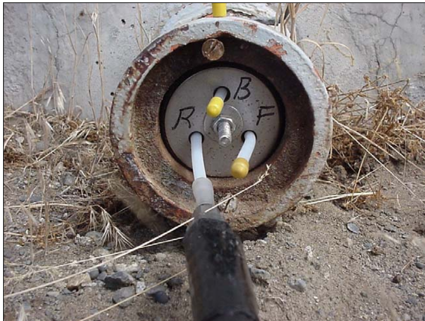
Figure 7. Storage Unit Drain Plug (Monitored Configuration)
