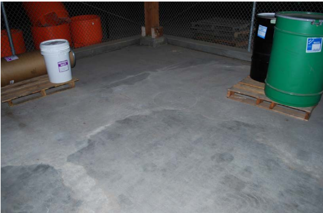
Figure 18. Building 203 CSF Battery Acid Spill Stain (Looking Southwest, March 2011)
