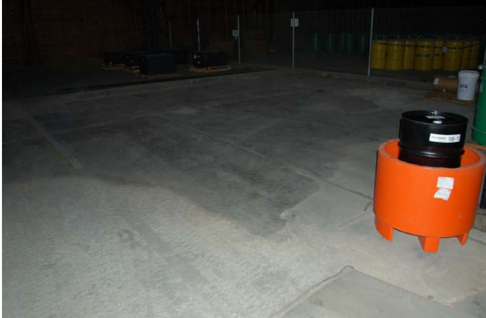
Figure 17. Building 203 CSF Battery Acid Spill Stain (Looking Southeast, March 2011)
