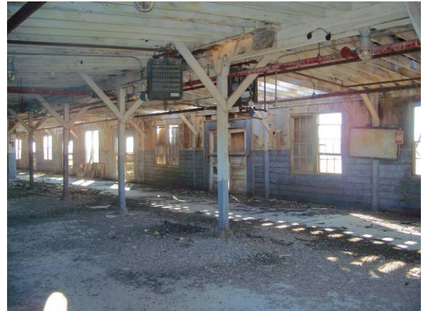
Less Than A Truckload & Boiler Plant Building (East bldg- inside)
