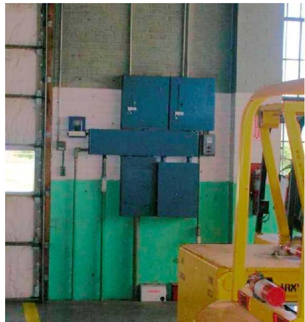
Old Main Breaker and Distribution Panel Eastside
