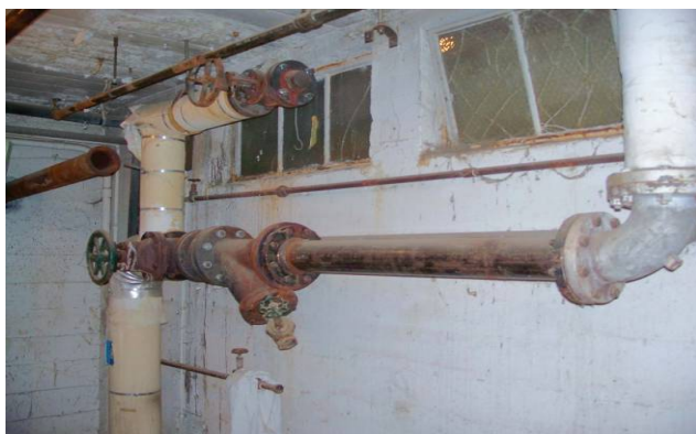
Piping Code Violation- Building 11 Basement
