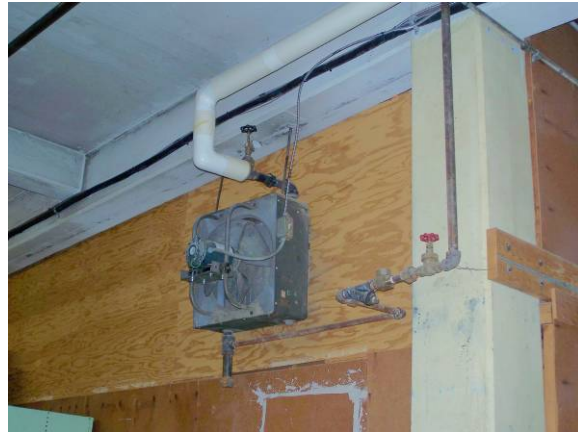
Typical: Admin Area Steam Unit Heater
