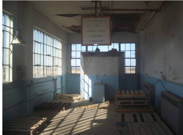
Surveillance Workshop (failing roof & insulation)
