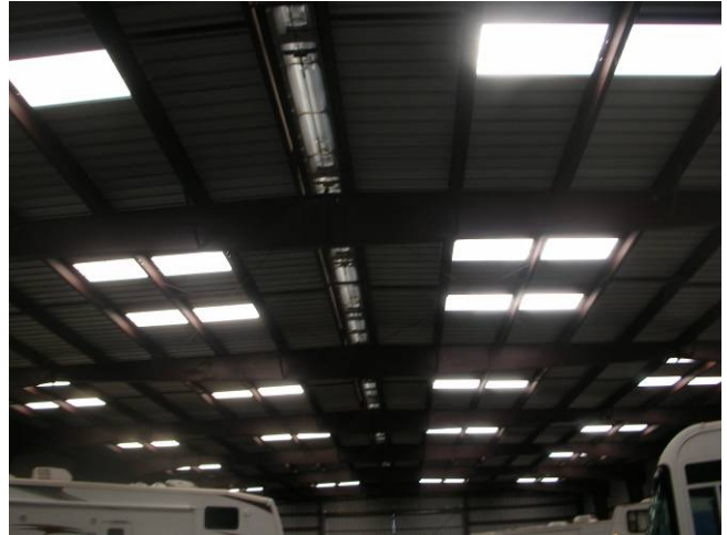
Bldg #450 (Skylighting only; automatic roof vents)
