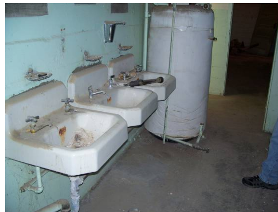
Plumbing Code Violation- Building 11
