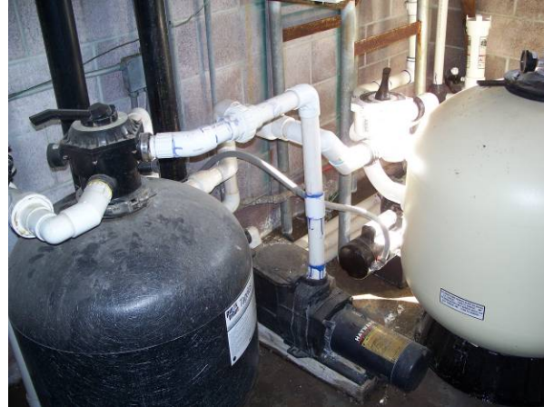
Pool Pumping & Filtration System
